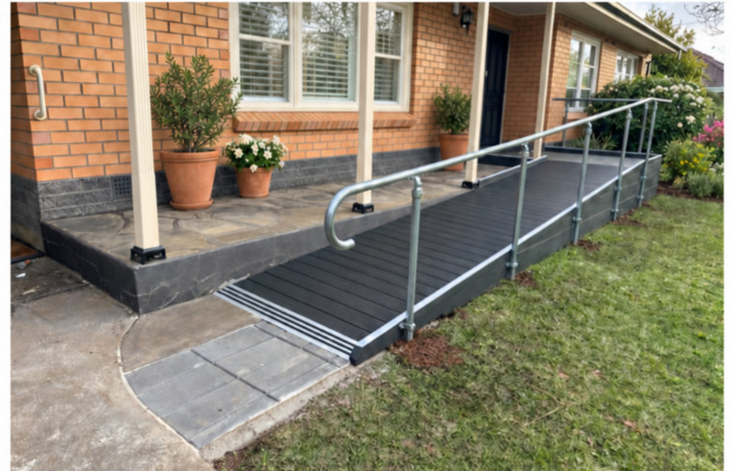
01 Full-length ramp and handrail system
